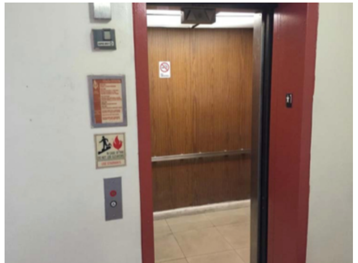
Elevator, fully wheelchair capable.
